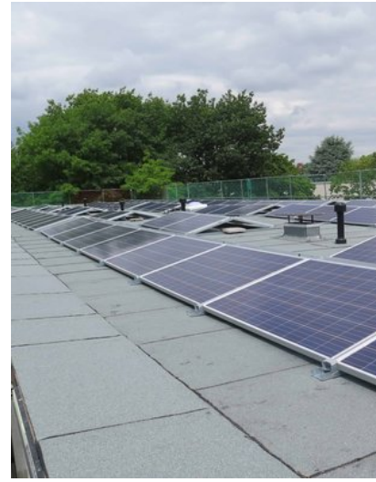
12 - PV system (example photo)
