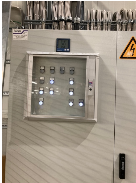
21 - Central control of the lighting
