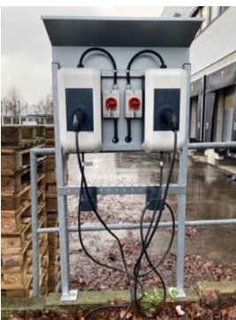
14 - Wallbox at the logistics site
